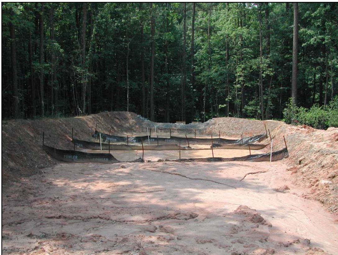
Figure 4. Standard trap with silt fence baffles (STSF) on 6 June 2005.
