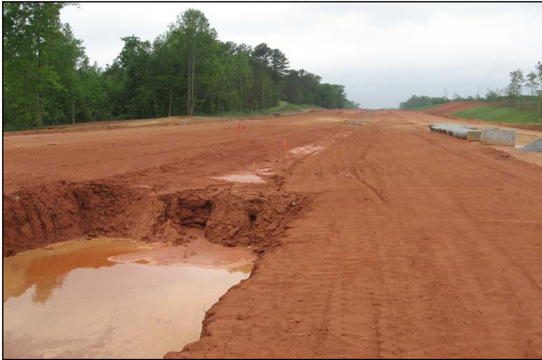
Figure 6. The STSP showing significant erosion at the unprotected inlet.
