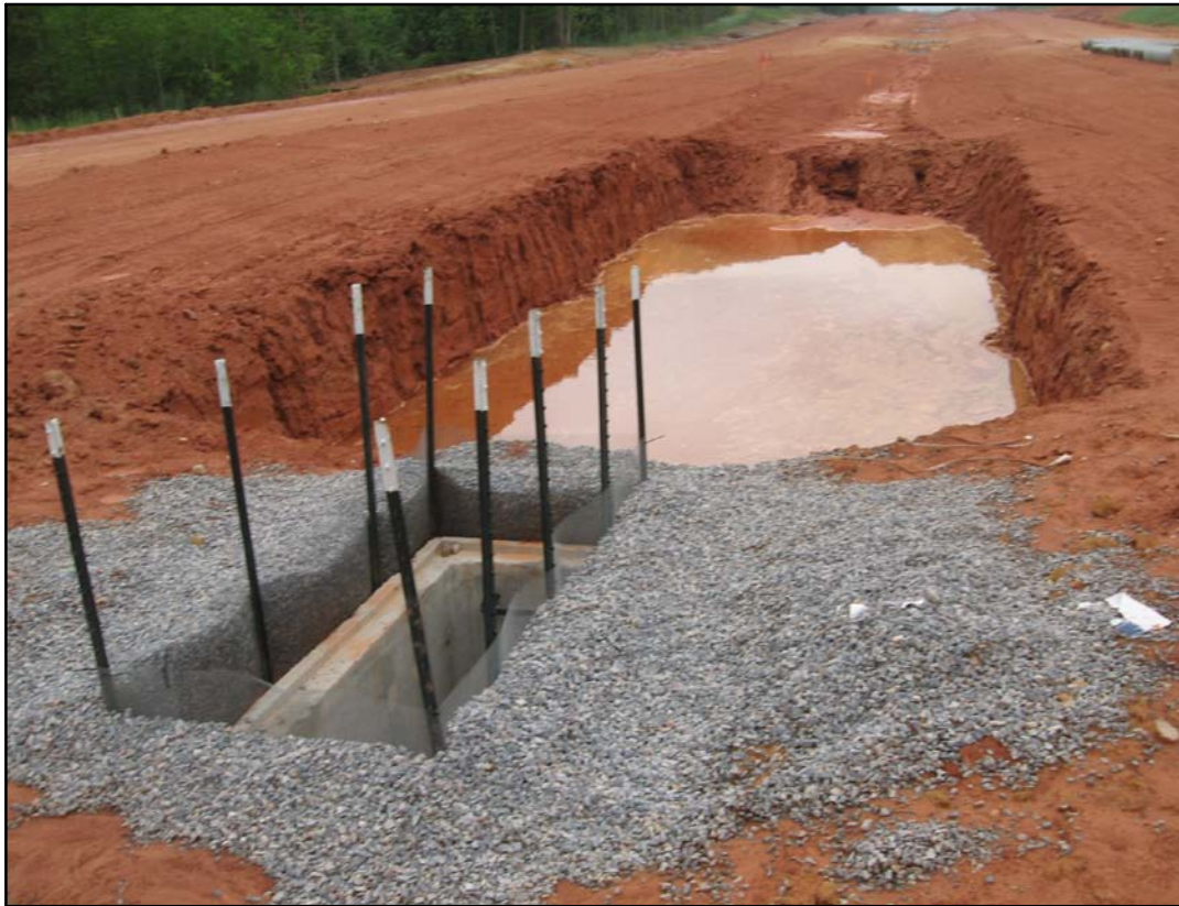
Figure 3. Standard trap with a standing pool (STSP) on 26 April 2006. Monitoring was conducted at the end of the pipe draining the drop inlet in the foreground.
